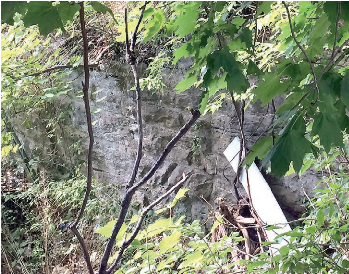
Limestone bridge abutment on the west side of Oatka Creek which is probably the Peanut line.
